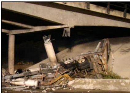
Figure 3: Impact damage of a bridge column
